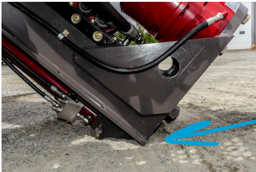
Figure 16 Mast completely flush with the ground.
